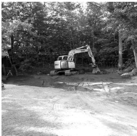
The cabins are down, and the space is ready for construction to begin.
